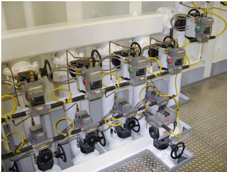
Figure 4: StoneL's FieldLink Bus Protection Module (BPM) works with AS-Interface to identify and isolate a short circuit in either the drop connection or on the main network "loop" allowing the rest of the devices to function normally. Used in conjunction with StoneL's Axiom valve communication and control monitor, BPMs improve safety by helping to prevent loss of process control. This reduces downtime and increases productivity.
